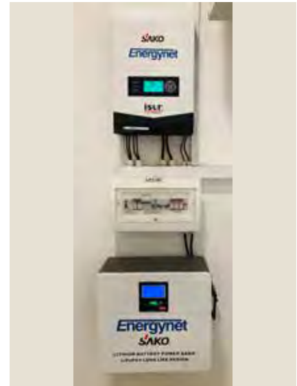
Solar energy system in place
